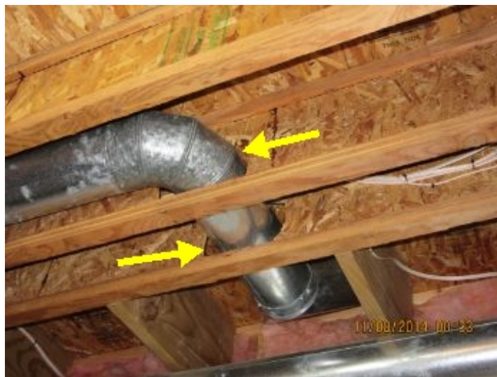
Improper holes in floor joists
