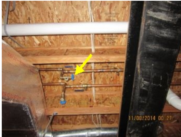
Leaking supply plumbing
