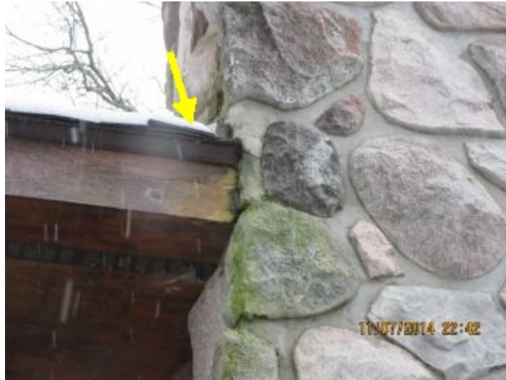
Review flashing at chimney
