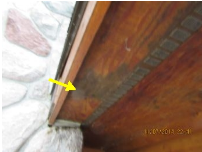
Warped soffit area at chimney
