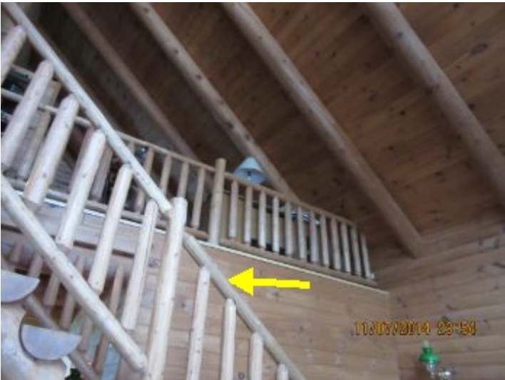
Unstable rail to upper level
